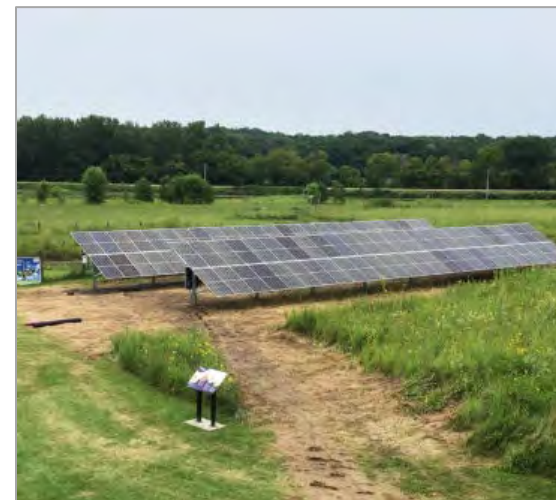
Solar array at Hurstville Interpretive Center. Photo Credit: Jackson County Energy District website
